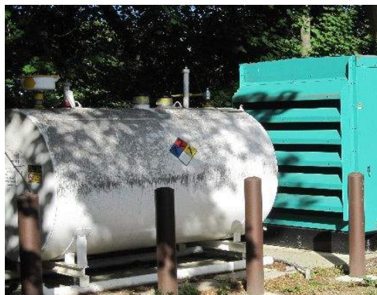
Figure 5-3. Fuel tank protected from traffic by cement posts.
