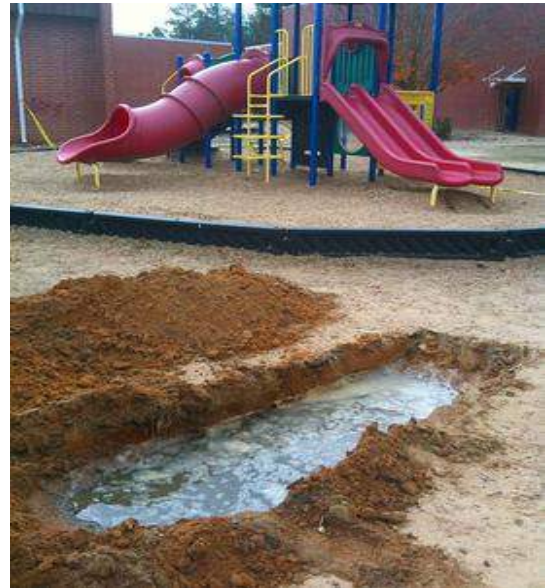
Failed septic system on a playground.
