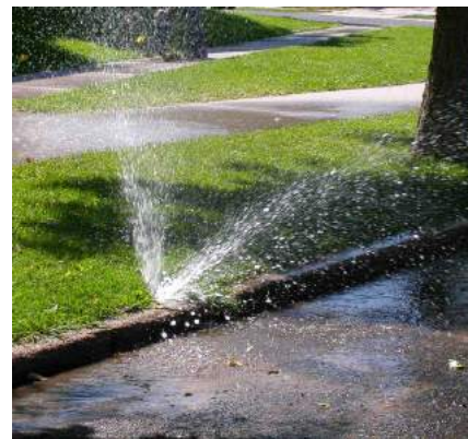
Figure 2-7. An improperly functioning sprinkler wastes water on street.
