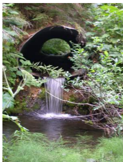
Figure 7-28. This culvert is too high. It creates a vertical barrier for fish and scours the outlet.
