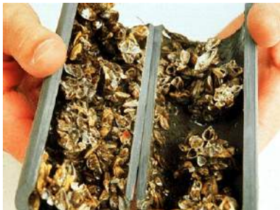
Figure 9-26. Clogged intake pipe.
