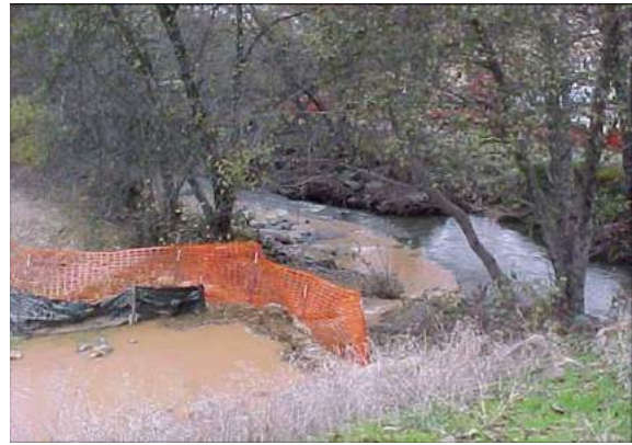
Figure 7-4. Poor placement of erosion control BMPs may result in sediments entering streams.
