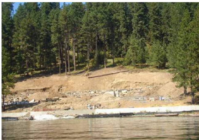
Figure 6-3. This building project does not provide an adequate setback from surface water.
