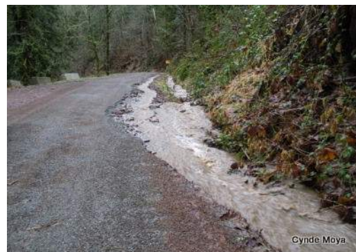
Figure 7-20. The result of an undersized/ clogged ditch.
