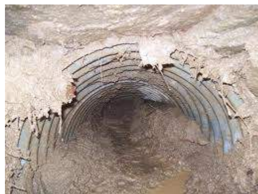
Figure 7-25. Culvert clogged with sediment.
