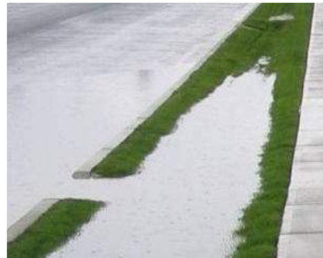
Curb inlet allows street stormwater to flow into grass infiltration system.
