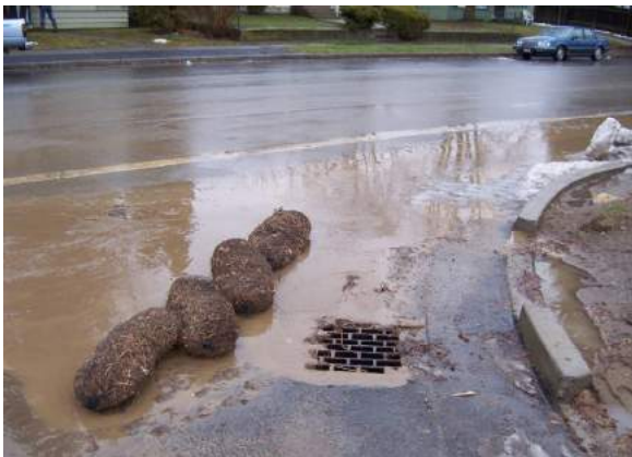
Figure 1-1. Improperly placed sediment controls allow polluted stormwater runoff into storm drain which flows directly to surface water.
