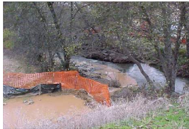
Figure 6-2. Improper erosion/sediment controls allow sediment to enter surface water.
