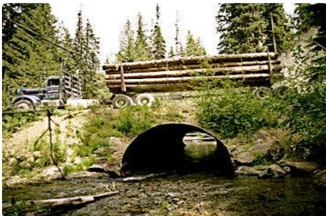
Figure 7-21. Fish-friendly arch culvert over a low-gradient stream.
