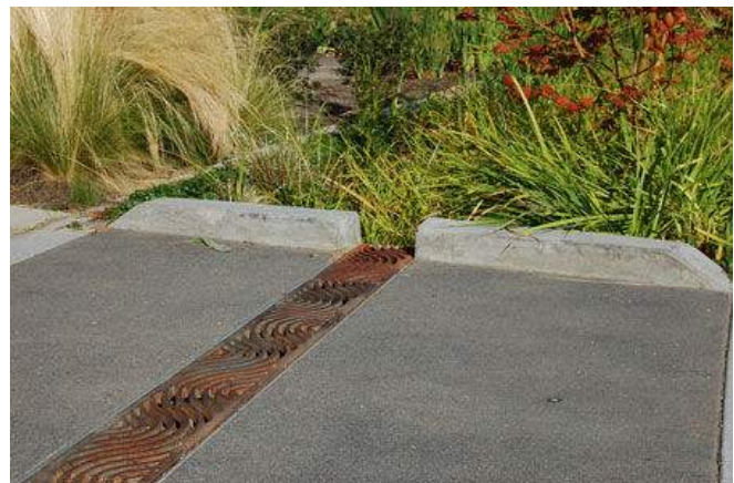
Figure 1-10. Decorative trench drain in driveway directs runoff to vegetative landscaping for infiltration.
