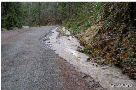
Figure 1-7. The result of an undersized/clogged ditch.
