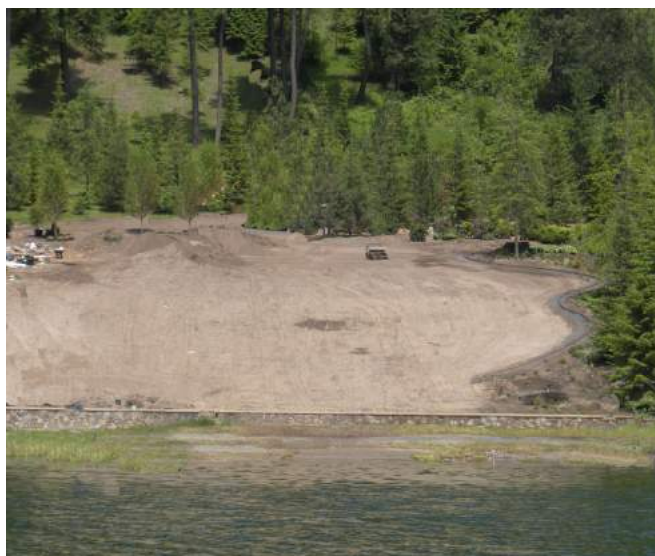
Figure 6-6. This project removed existing vegetation near the shoreline and exposed bare soil to stormwater and wind.
