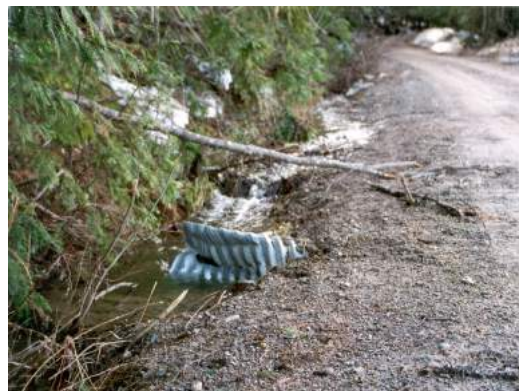
Figure 7-7. Crushed culvert cross drain.
