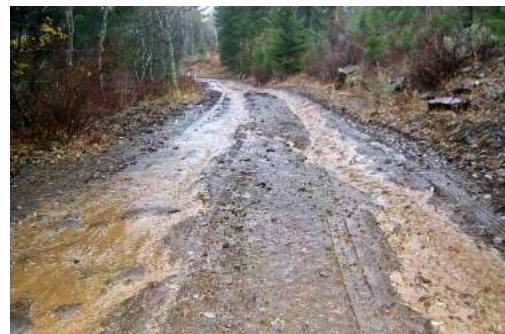
Figure 7-1. Improper grading and drainage creates ruts and gullies in roads, increasing erosion and sedimentation.
